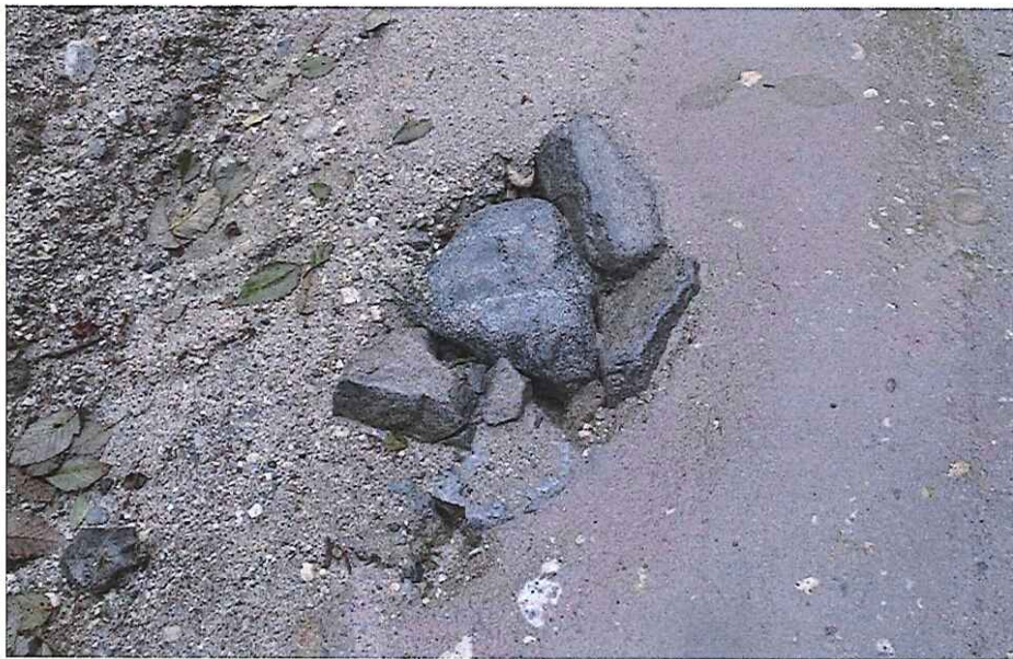
CK2267 Deck Damage
